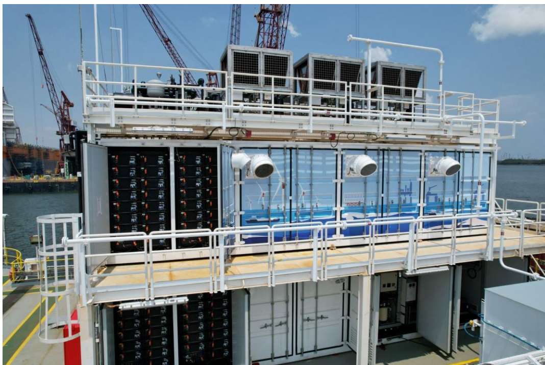
Photo of Southeast Asia's first floating and stacked Energy Storage System, with maximum storage capacity of 7.5 megawatt hour (MWh) to power over 600 four-room HDB households in a single discharge. (Photo credit: Seatrium Limited)
