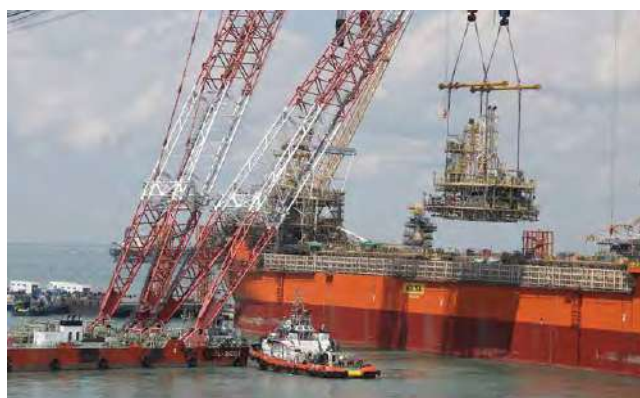
Topsides installation on a floating storage and offloading vessel which will be deployed at the Culzean field
