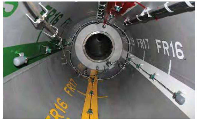
EIMag installations onboard a tanker fleet operating in the environmentally-sensitive US Alaskan region
