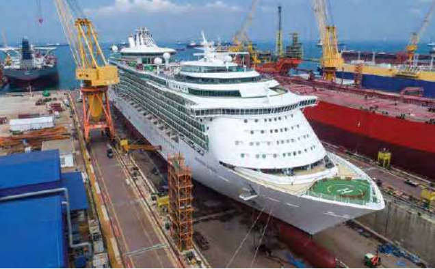
Royal Caribbean International's Mariner of the Seas revitalisation project at Tuas Boulevard Yard
