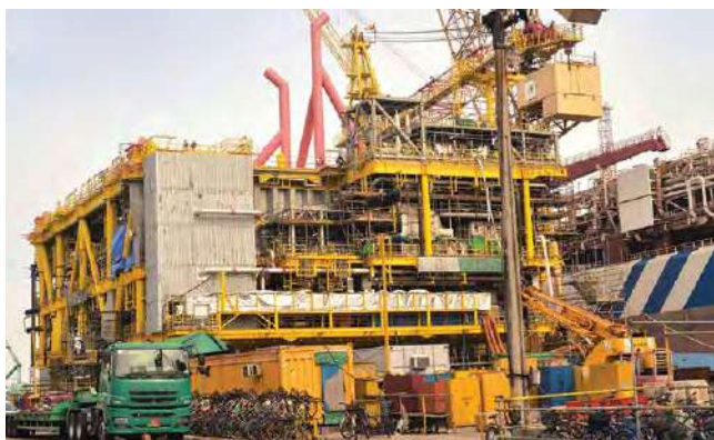
Maersk Oil's Wellhead Platform topside
